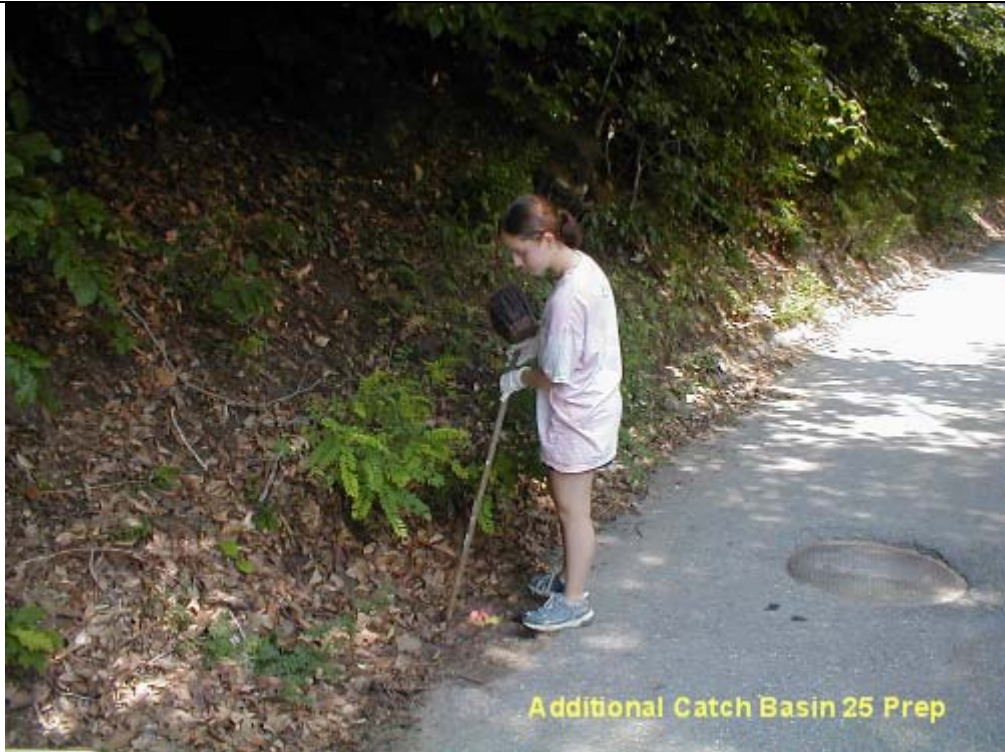
Using a stick or a broom or rake handles all dirt and debris blocking the catch basin was removed
