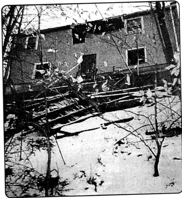
Fig. 10.1 Above: This house at 228 Lakeshore Drive had to be totally rebuilt, including a new foundation. (construction and photo by Bud Carrier, 1985)
